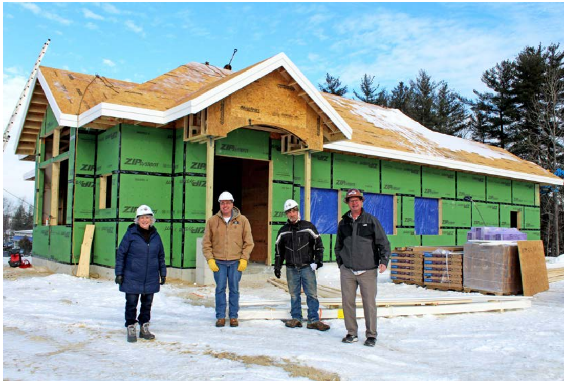
Project managers, including MVSb's Alison Whynot, Vice President of Facilities, and Thomas Cimikoski, Facilities Manager, give a tour of the Rochester construction site.
